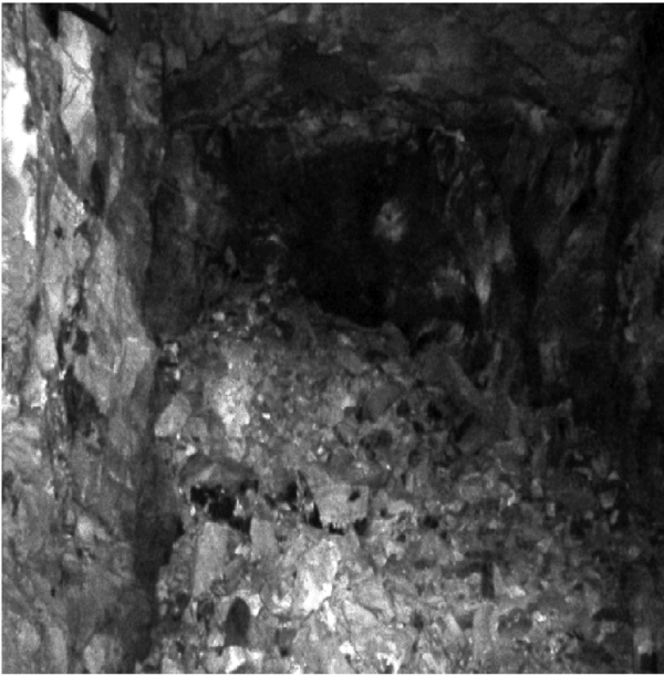
Fig. 10. Fracture zone at the inserted quartzite layer of Eunsan gold mine.
